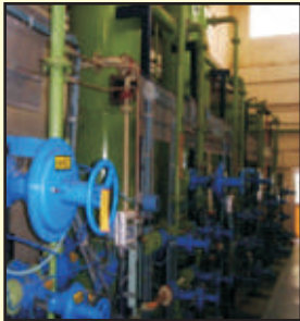
DM PLANT INSTALLED 2 x 15 m 3 /hr, 3 x 45 m 3 /hr, 3 x 15 m 3 /hr, 2 x 7.5 m 3 /hr
