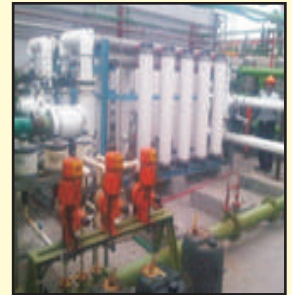
UF SYSTEM 2 x 140 m 3 /hr
