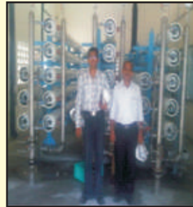
RO PLANT 2 x 120 m 3 /hr
