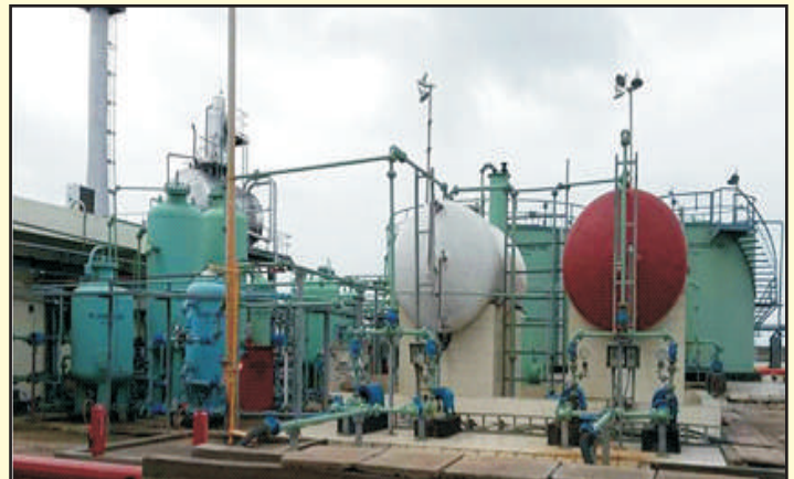
DM PLANT, CPU AND Effluent treatment plant renovation at IOCL, LPG Import terminal , Kandla,Gujarat.
